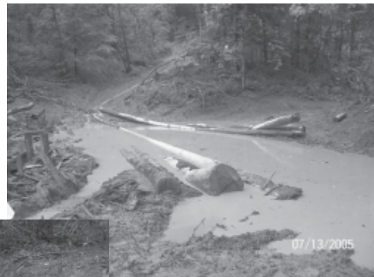
Above: Skid trail running downhill into flat next to stream. Notice flow of muddy water coming down skid trail from uphill seep. Water bar or other water control was needed to divert this flow before it gets to the bottom next to the stream.
